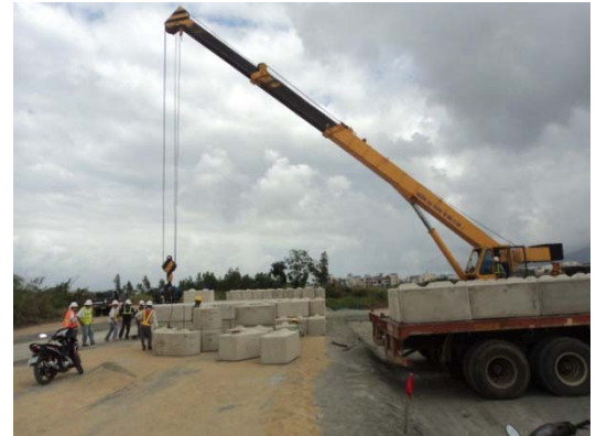
Constructing walls of the pile containment structure with CMU blocks (Photo: CDM Smith)
